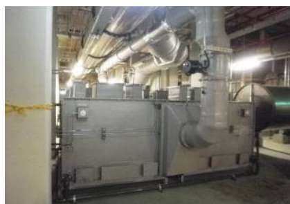
除臭觸媒吸附塔 Deodorization Catalyst Adsorber
