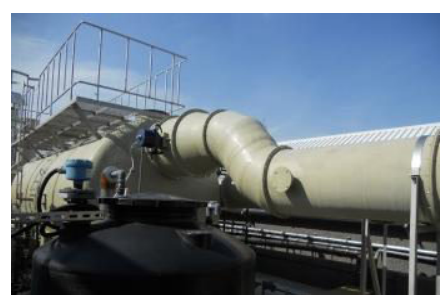
除煙除酸除臭觸媒吸附設備 De-smoke, de-acid and de-odor equipment
